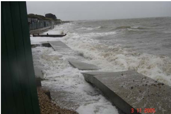
Figure 1. Storm damage at Hill Head (Photo: D Watkins)
