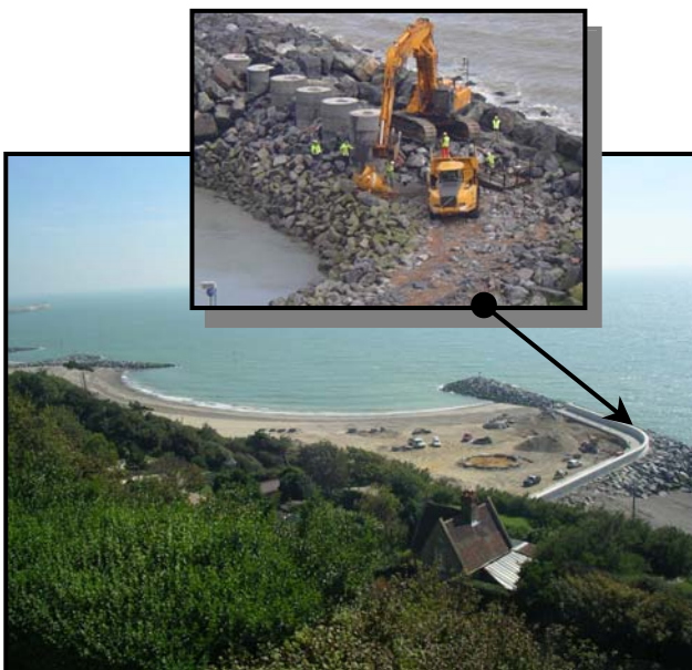
Figure 1. Photographs to show the construction phase and completed scheme at Folkestone, Kent
